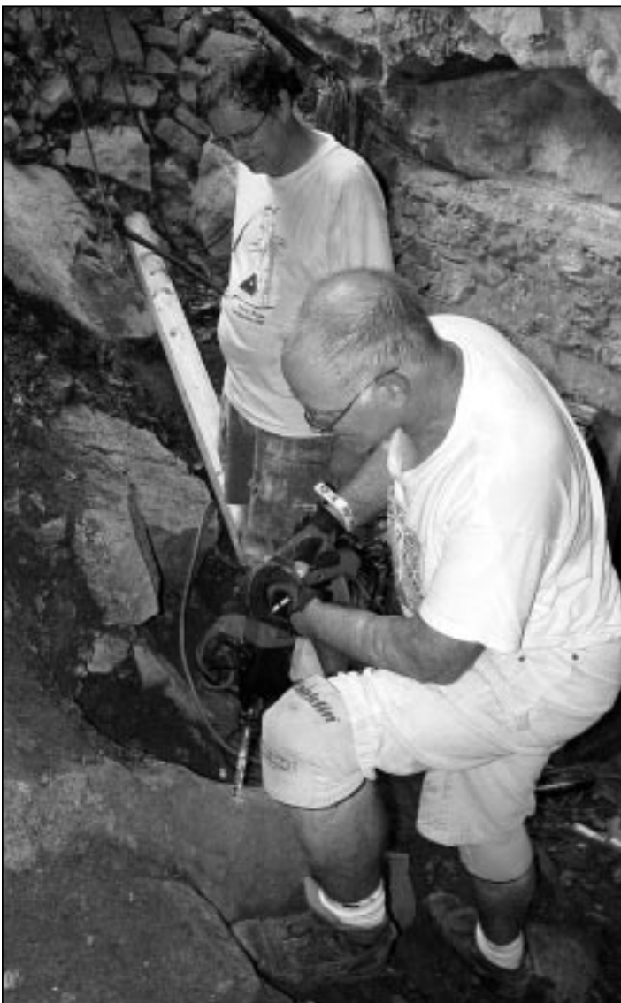
Joe Jones & Grayson Knapp constructing a handrail at the cave entrance. Photo by Geary Schindel.
